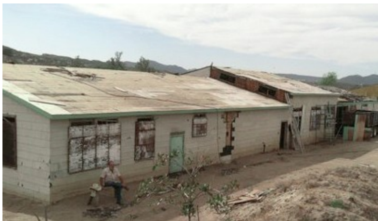
Camp Lockett building 605 with the old roof showing years of weathering. MTM volunteers will remove the old roof, restore the underlayment and then the roofing contractor will install the new green roofing material.
